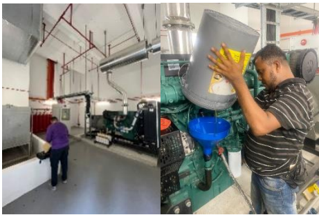
Monthly Servicing of LV System, Transformer and Genset Room
