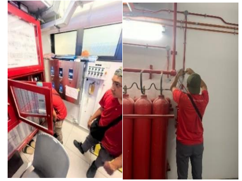
Fire Equipment Servicing
